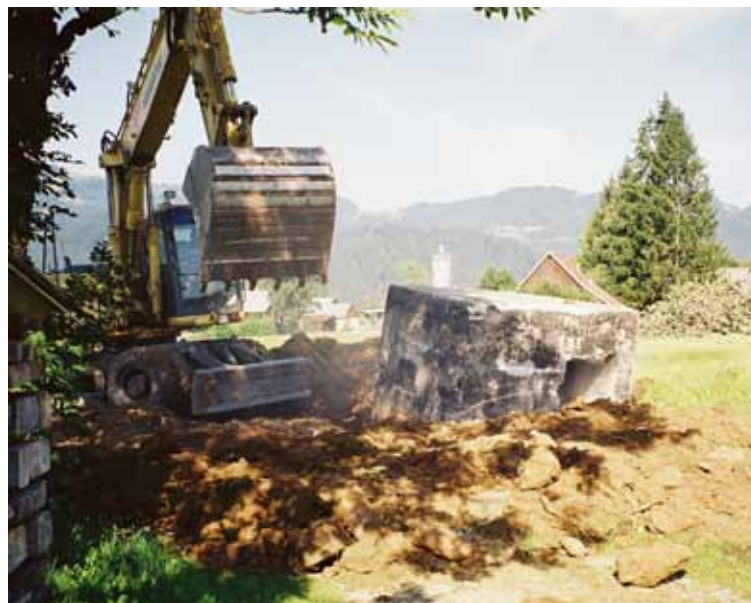
Figure 4: Until 18 September 2007 the bunker stood at the end of the street Pot na Koče. It was removed by Anica Likovič when the the road to the “Grugatova” house was built. It is now buried in the construction pit underneath the previous dirt road (author of the photograph: Zvone Kopač, 2007; source: author’s archives).
